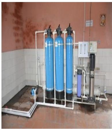
RO PLANT AMRAPALI
