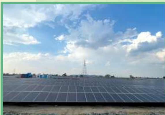
View of Solar panel at Piparwar Area
