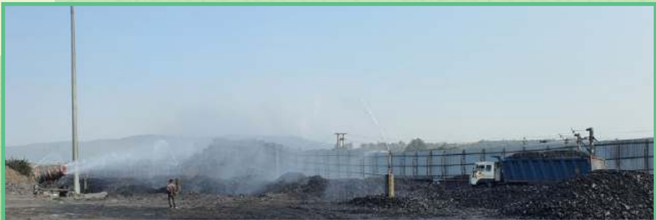
View of fixed sprinkler at North Urimari
