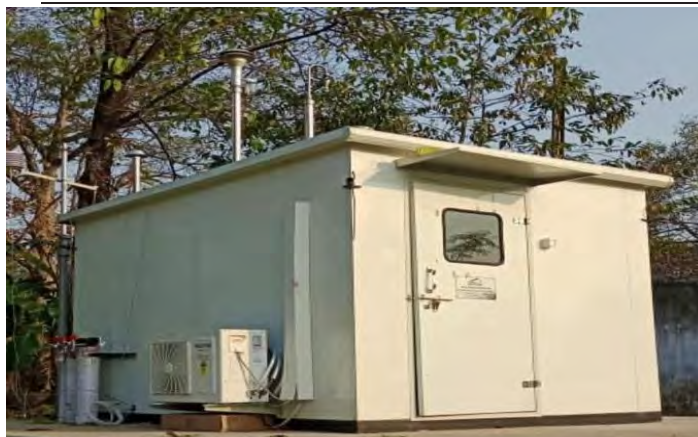
Installed CAAQMS at Bokaro & Kargali Area of CCL
