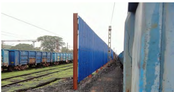
Wind Braking system at Piparwar & RCM Railway Siding of Piparwar Area
