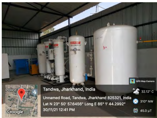
Oxygen Plant Chatra
