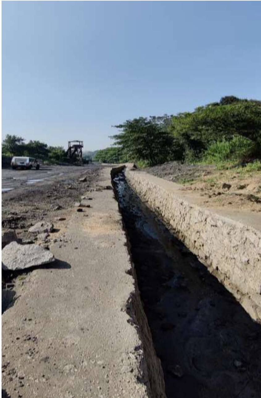
Figure 1.11 Drains in Dakra Mine
