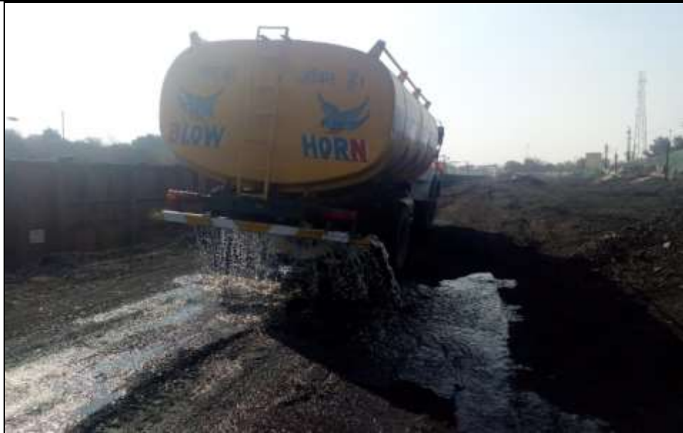
Figure 1.4 28 KL Mobile Sprinkler Mobile water sprinkler at Dakra siding
