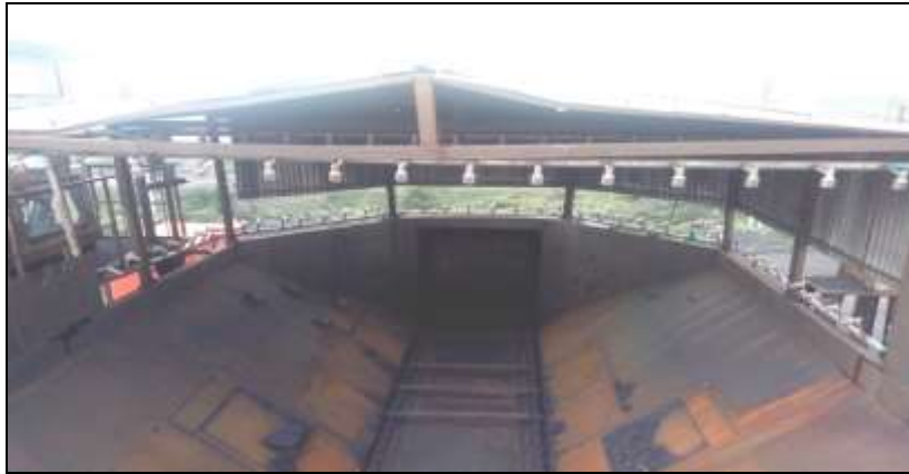
b) Covered Feeder Crusher with water sprinkling system (August 2018)
