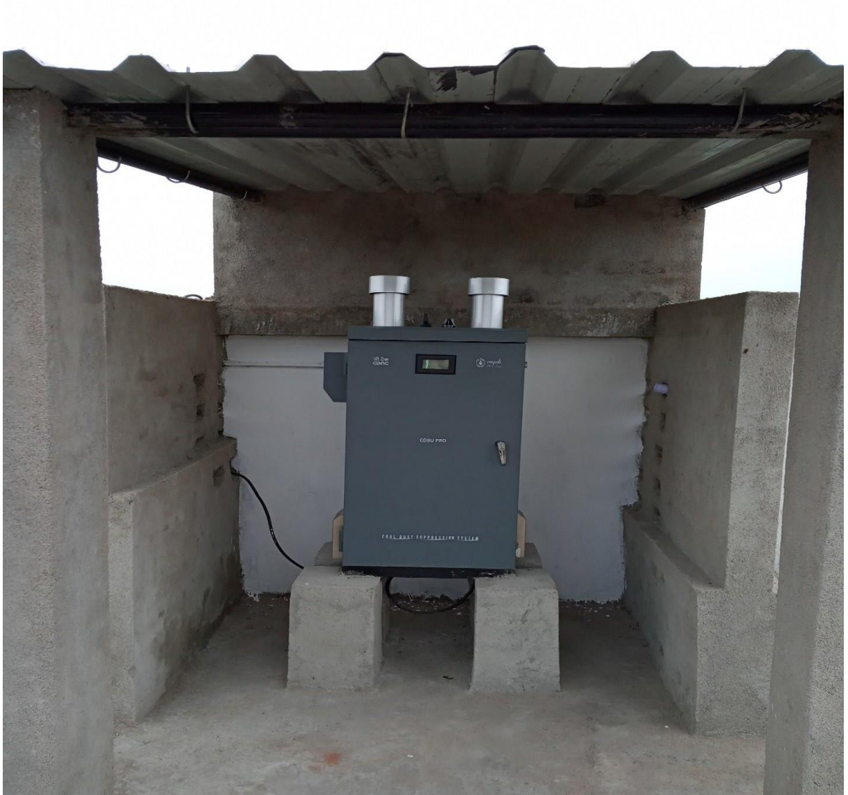
CAAQMS AT RCM SIDING ASHOK OC PROJECT, PIPARWAR AREA, CCL.
