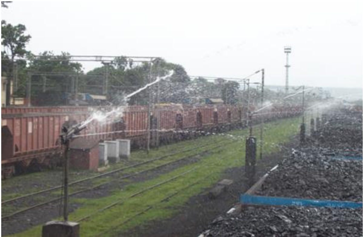
FIXED SPRINKLERS AT RCM SIDING ASHOK OC PROJECT, PIPARWAR AREA, CCL.
