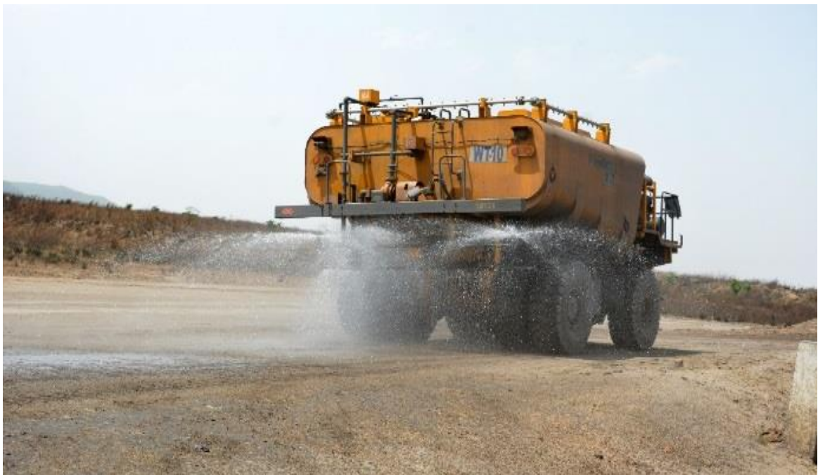
MIST SPRAYERS AT ASHOK OC PROJECT, PIPARWAR AREA, CCL.
